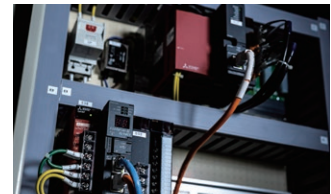
EcoWebServer III installed on-site (bottom of photo). Above is a PLC for collecting data from measuring instruments.
