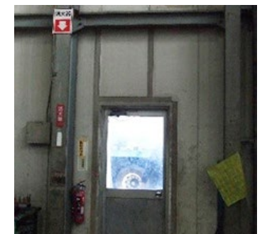
Doorways and evacuation routes (Gunma Works)
