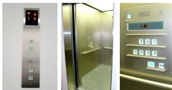
Barrier-free elevator (Advanced Technology R&D Center)
