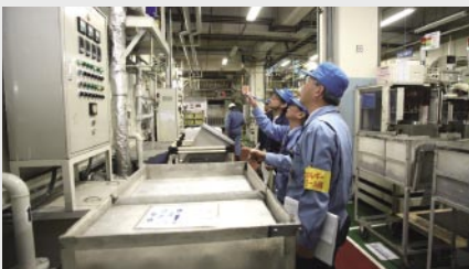
This steam heater is being used for heating, but it is inefficient due to significant steam loss. Since the temperature is low, you should be able to use a more efficient heat pump.
