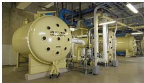
Ozone generation equipment
