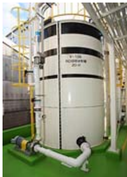
Recycled water storage tank.
