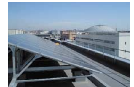
Nagoya Works (FA R&D Center) Photovoltaic power-generation system panels mounted on rooftop.
