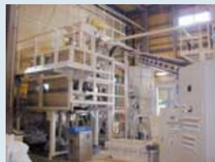
Plastic separation system
