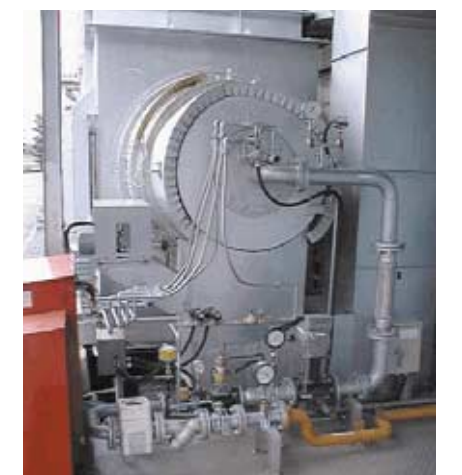
Deodorizing equipment burner section after shift to city gas.
