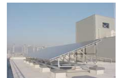
Communication Equipment Works Photovoltaic power-generation system panels mounted on rooftop.
