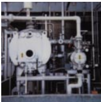
Waste Alkali Evaporation and Condensation System
