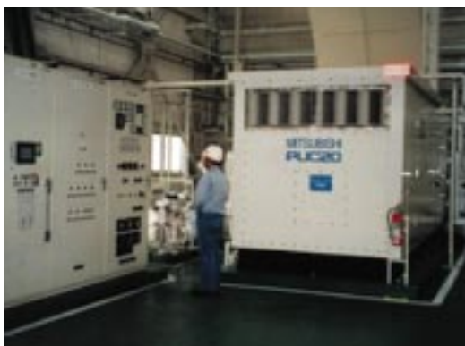
Gas Turbine Co-Generation System
