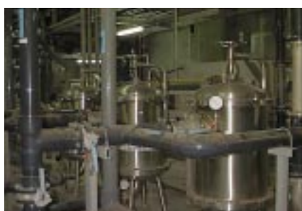
Liquid Waste Recycling System
